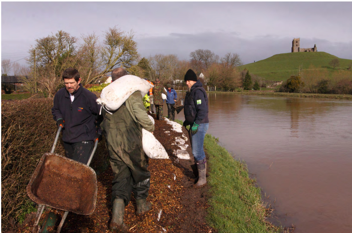
Figure 5. Volunteers act to reinforce a footpath along the banks of the river Parrett, Somerset, February 2014 (Steven May/Alamy Stock Photo)
